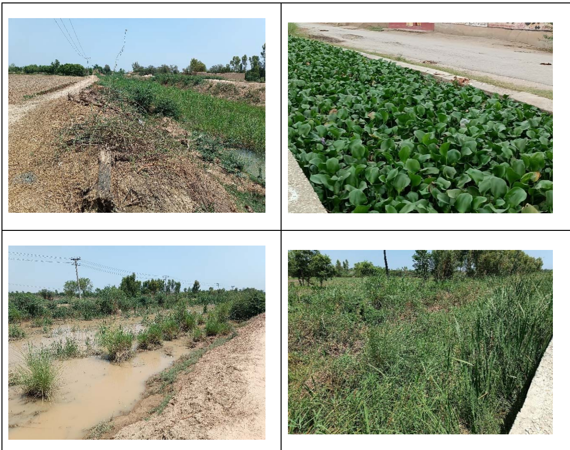
Figure 1.4: Heavy Silt, Vegetation and Sarkanda in Drains
